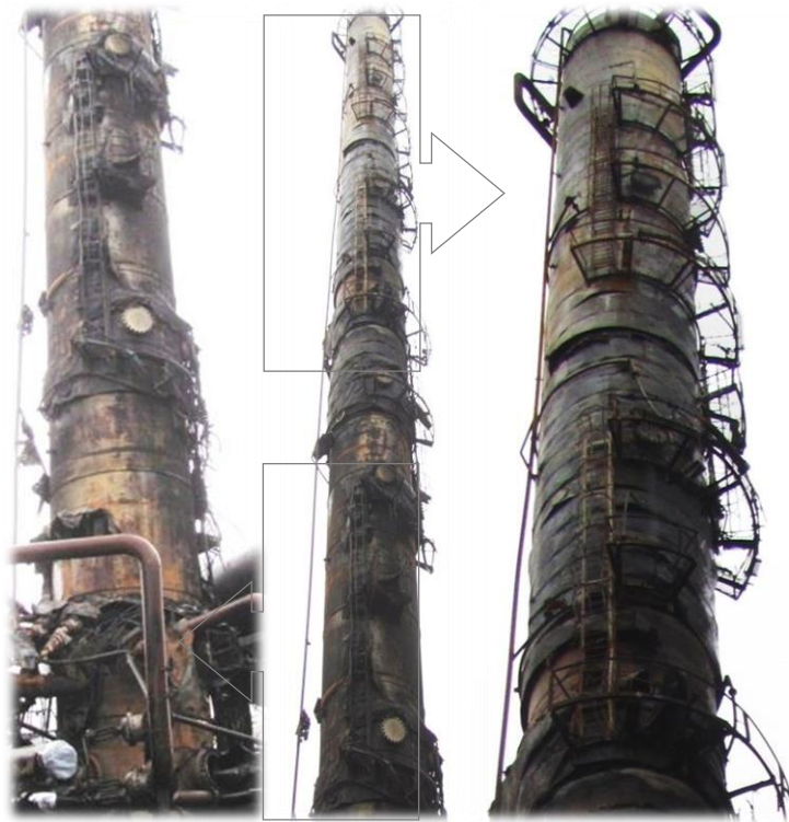
Fig. 2. The rectification column after the accident
